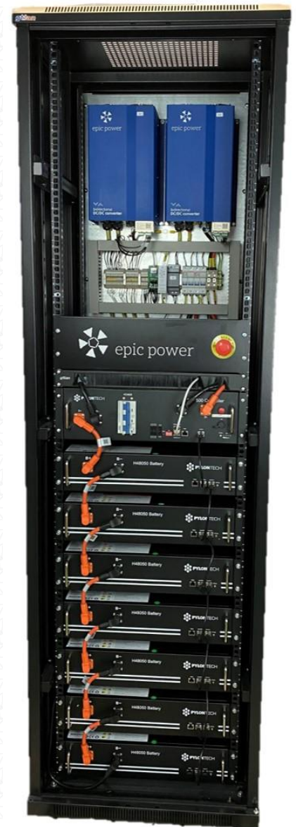
Fig. 6: Plug&Play solution in existing installation. LiFePO4 + DC/DC converter
